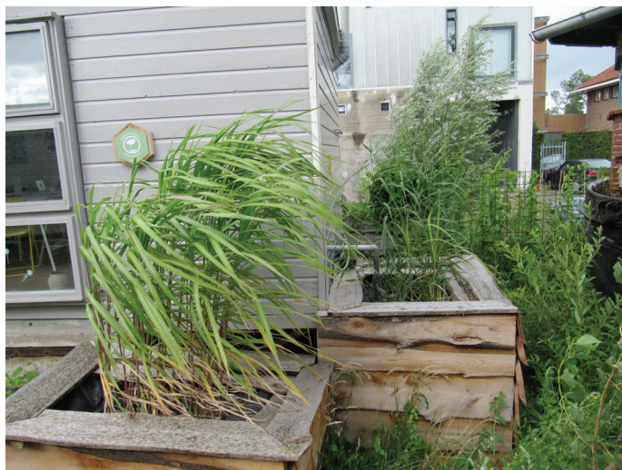
Fig. 2. Grey water treatment in individual low-tech biofilters, consisting of two IBC containers filled with layers of gravel and coarse and fine sand, planted with reeds.
